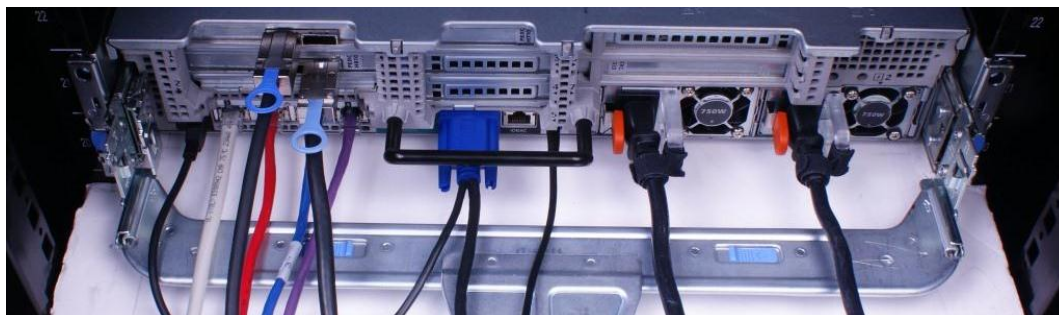
Figure 1. System with cables installed
